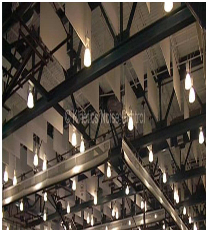
Noise control baffles (fiberglass)
