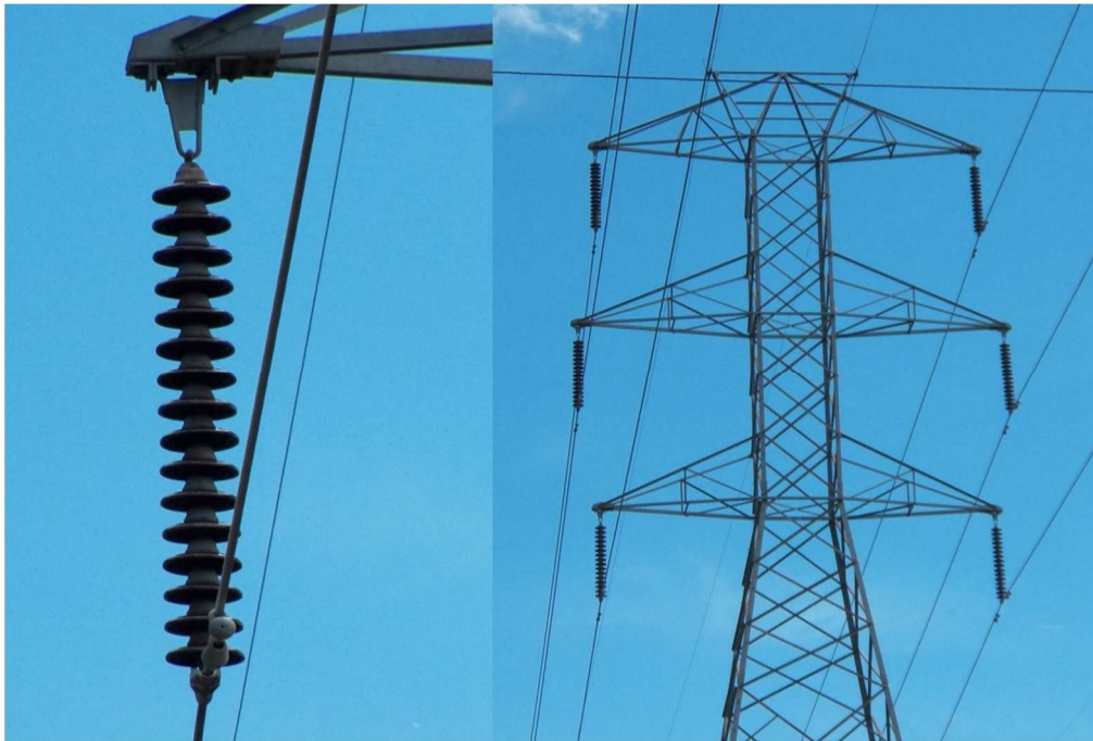
Figure (4.7) Overhead transmission lines
